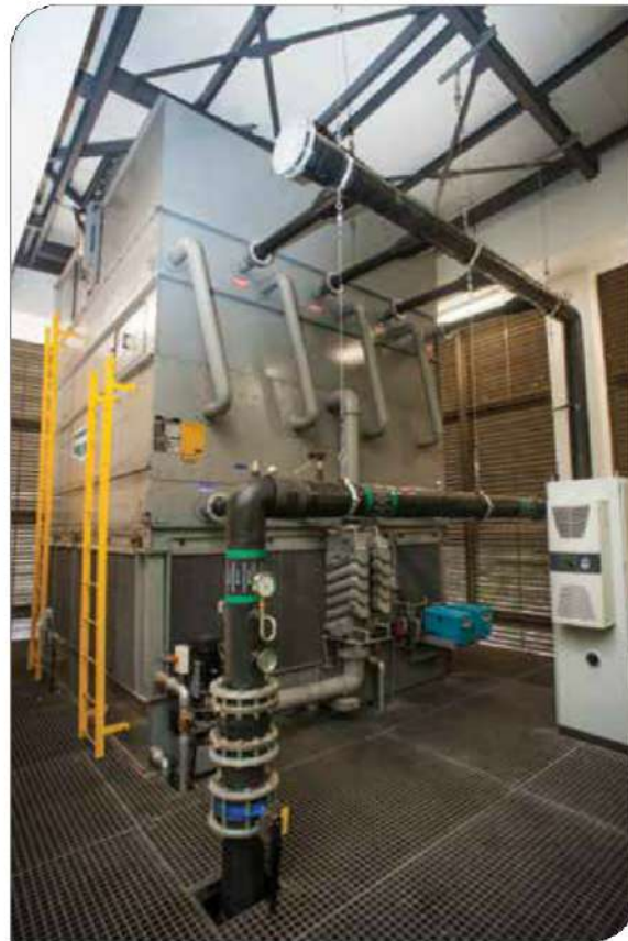
Hybrid Evapco cooling tower. Note the grid – there is a 1m deep access floor where all pipes are hidden.
